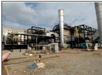
Total Lacq France - 30 MWth Oxy - Gas/Fuel
