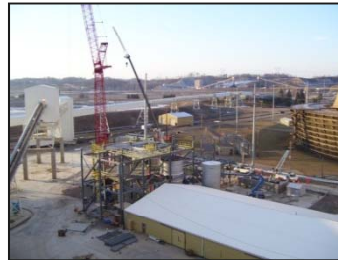
AEP Mountaineer USA - 30 MWth Chilled Ammonia - Coal
